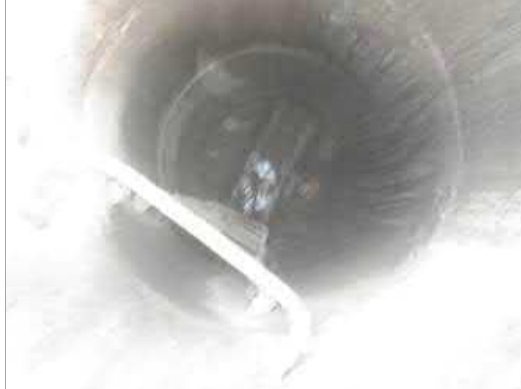
MH Top View Photo
