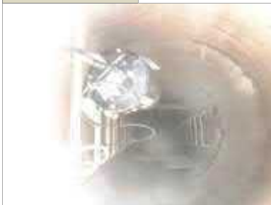
Flow Meter Installation Photo
