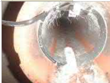
Sensor Installation Photo
