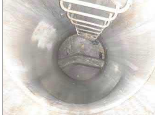
MH Top View Photo
