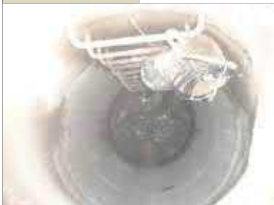
Flow Meter Installation Photo
