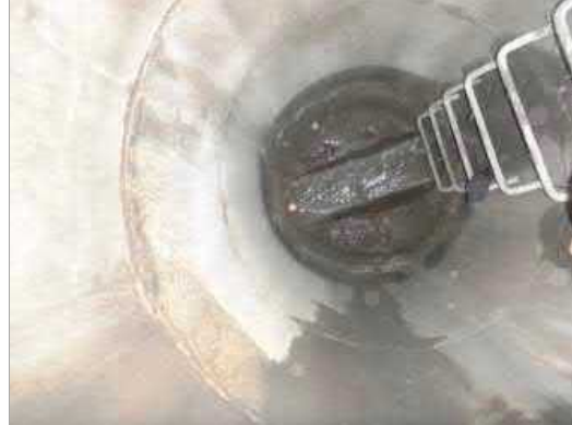
MH Top View Photo
