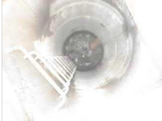
MH Top View Photo
