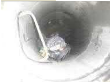
Flow Meter Installation Photo
