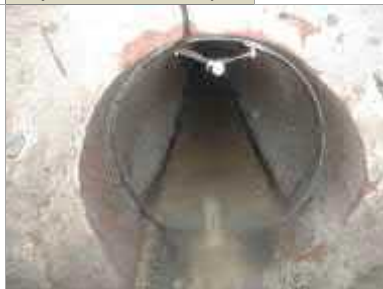
Sensor Installation Photo
