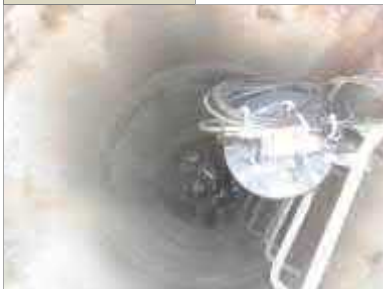
Flow Meter Installation Photo
