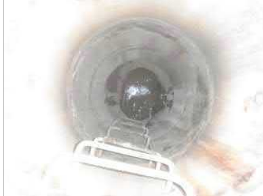
MH Top View Photo
