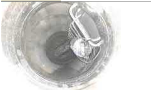
Flow Meter Installation Photo
