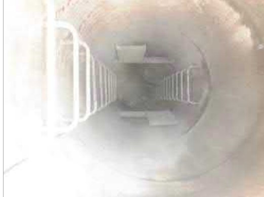
MH Top View Photo
