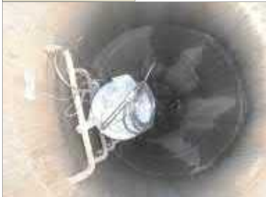
Flow Meter Installation Photo
