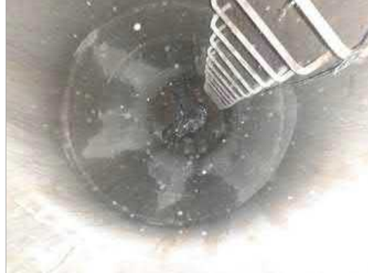
MH Top View Photo
